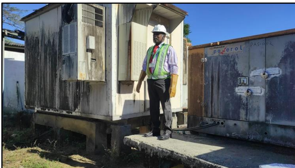
Energy conservation facilities observed in the Campus
